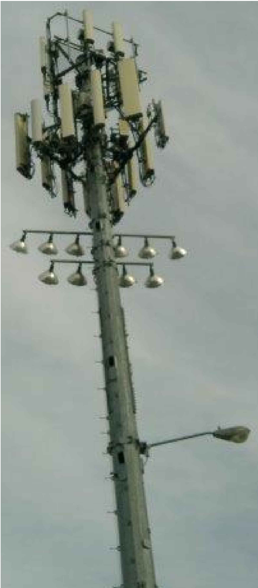
PHOTO OF EXISTING TOWER
